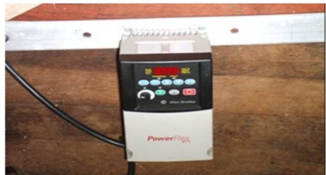
Fig. 5 Shows the power supply to heat injection fan.
