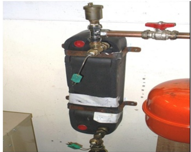
Fig. 2 Shows the heat exchanger.
